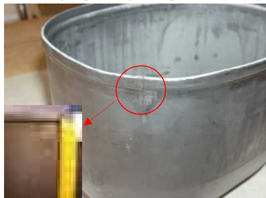
Fig. 1. Crack on the compressor cover
